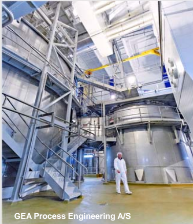
GEA Process Engineering A/S
